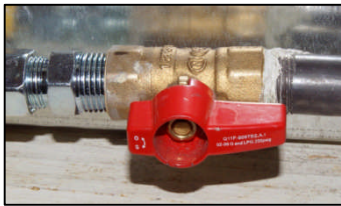
Gas Shut-off Valve
